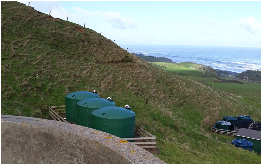
MOKAU WATER SUPPLY - NEW STORAGE TANKS
